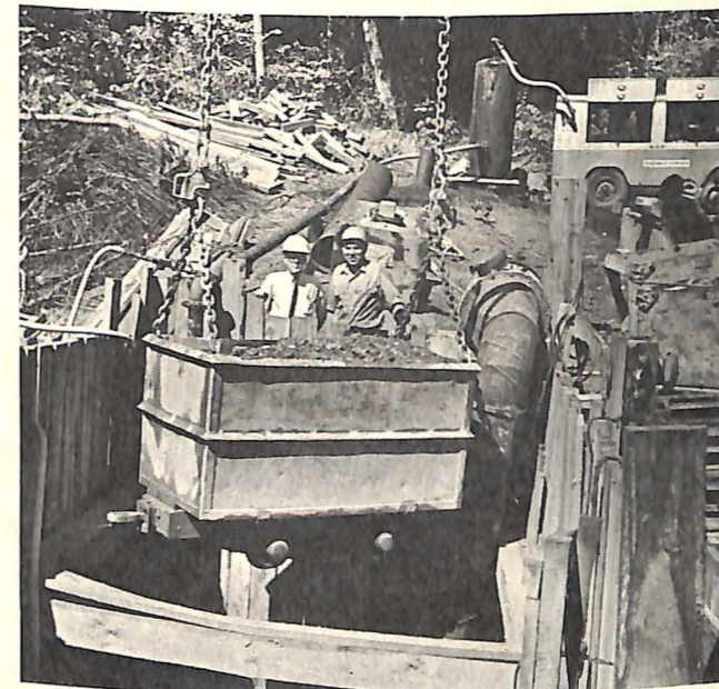
Material being removed from the tunnel area. Individuals shown in photo are: Sam McGhee, City Engineer, and Al Greenwood, Project Superintendent for McHugh Construction Company.
