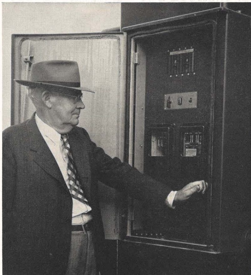
Howard R. Collins, former Ashland District distribution superintendent, energizes the new Ashland substation which was named for him.
