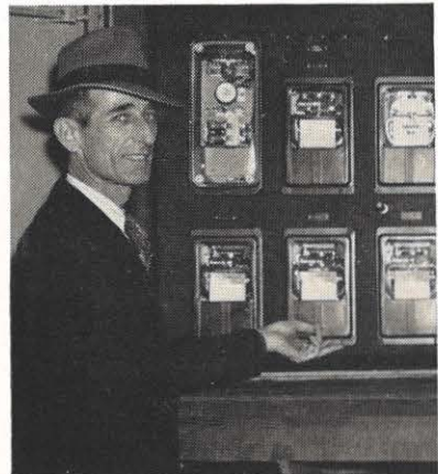
George E. Hervey, Charleston district substation superintendent, is shown at the control panel of the mobile substation during a routine inspection in Charleston.
