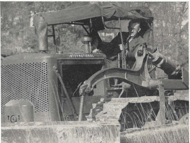
Work is under way on the new substation being built in Bluefield. District Manager L. W. Bates was at the scene of the new substation when the first shovel full of earth was moved. Here he tries his hand at a bulldozer.
