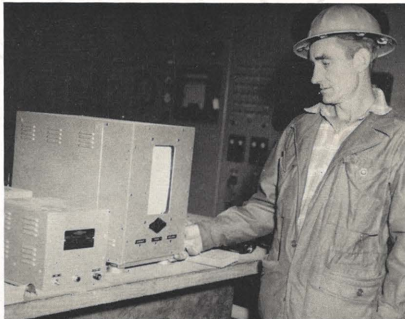
C. R. Tennant, assistant shift operating engineer, checks the television receiving set before it is installed in the control room at the Sporn Plant.
