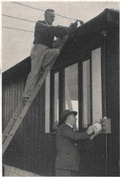
J. A. Randall, meter superintendent for Kingsport Utilities, installs the meter for the 16,000th customer served by the company. Helping to install service is W. D. Trent on the ladder.
