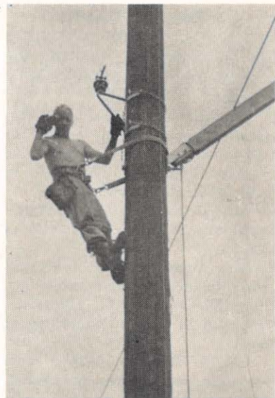
R. A. Walk, system transmission department uses his "handie-talkie" radio at a high check-point during a conductor-pulling operation.
