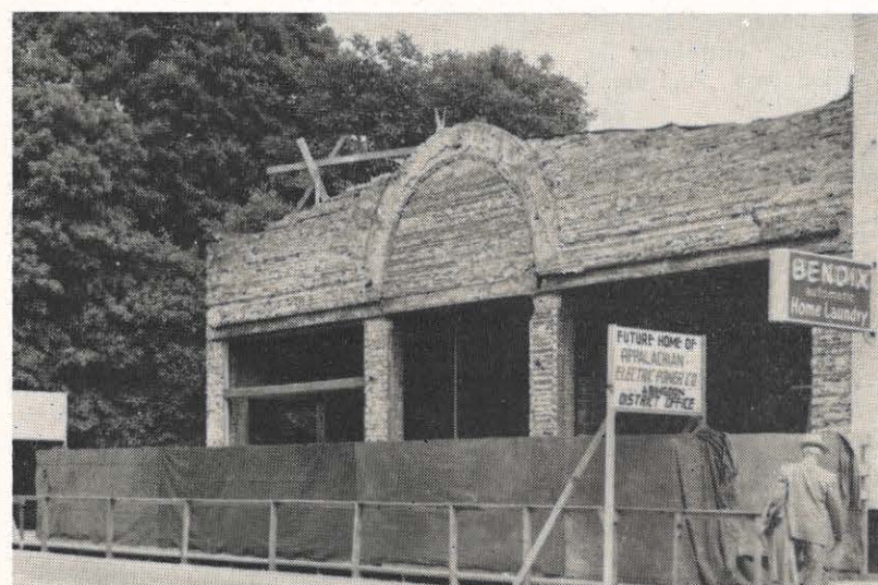
Shown above is the Abingdon district office building as it is undergoing an extensive remodeling. The property was formerly owned by the Abingdon Motor Company.
