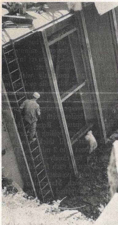
Workmen shown above are working on the trash screens at Niagara plant. The man on the ladder is checking the new screen while the other workman shovels muck away from the base of the screen housing to leave room for another screen.
