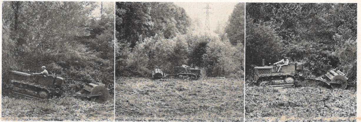
Shown above are three pictures of the equipment which W. P. Carter, system transmission line superintendent, designed for clearing rights of way. The article on this equipment and its use was awarded first prize in the annual A. G. and E. Monthly Operating Notes contest. In the picture at the left, the tractor is shown being used in a forward motion to wreck some of the undergrowth. The center picture shows the condition of a right of way after it has been cleared by the tractor and drum. The picture at the right shows the tractor in reverse motion and the action of the drum in clearing the right of way.
