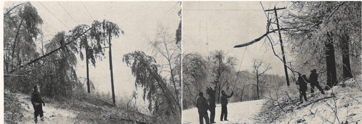
The weatherman played these tricks in at least two districts of the company last month. The photo at the left shows an Ashland district employee clearing the limb of a tree from a high voltage line. In the photo at the right a Huntington district line crew removes the branch of a tree from a distribution line.
