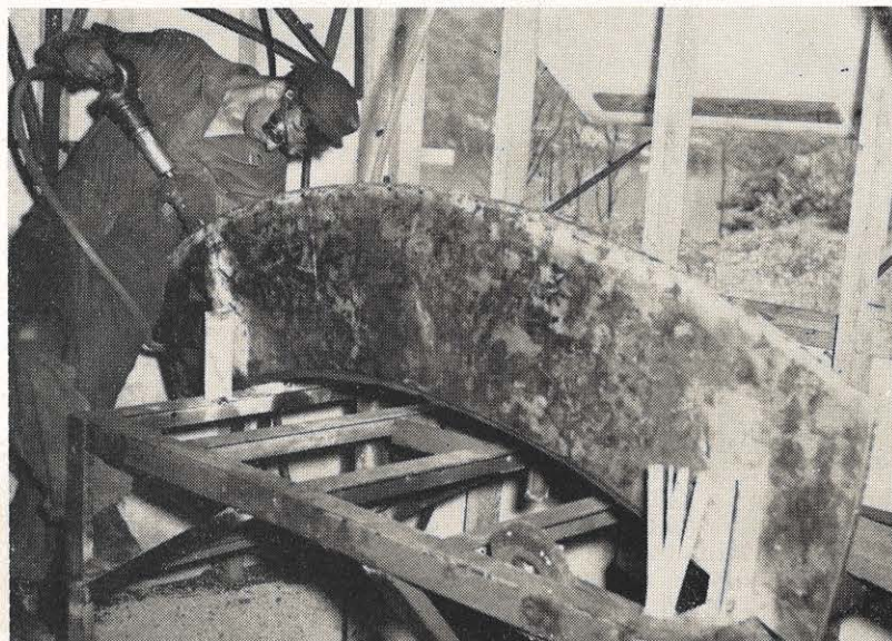
The welding, reshaping and grinding of all blade tips was done in the shop, accounting for the 50 per cent savings in the new method. The workman above is peening a weld on the outer edge of one of the blade tips which has been coated with stainless steel.
