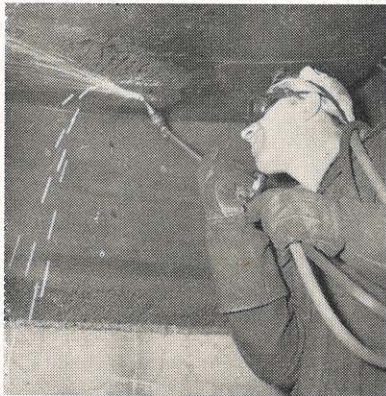
Doing the work with a gouging nozzle in 30 minutes that used to take eight hours with a chipping hammer, the workman above is cutting out a pitted section on the water wheel blade. Another pitted area can be seen on the throat ring on the man's right.
