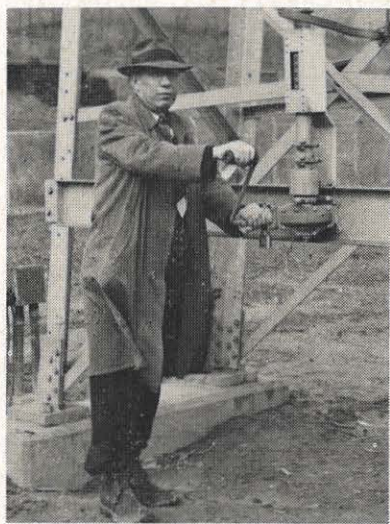
Charlie McKinney, Pikeville district superintendent, is shown closing the switches of the new 132 kva substation at Betsy Layne, Ky., March 9. Betsy Layne is equipped with 20,000 kva transformer bank which is tied to the Sprigg-Beaver Creek Number 3 line. It provides the Pikeville district with an additional source of power.
