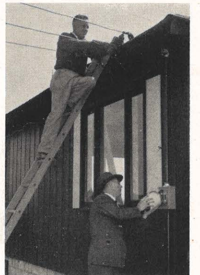
The 16,000th customer of Kingsport Utilities was connected in April, 1950. In the photo below, Kingsport employees are shown connecting the service to that customer.
