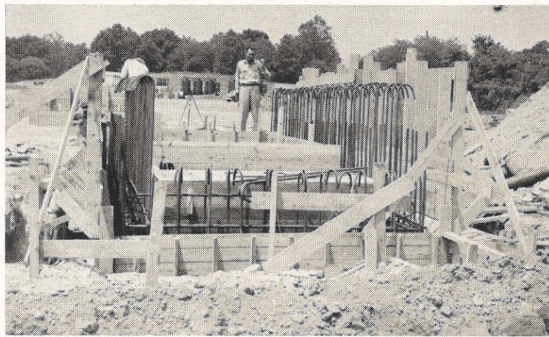
Foundation work at Hancock nears completion. In the photo above, workmen ready forms before pouring concrete for the foundation of the 100-ton synchronous condenser.
