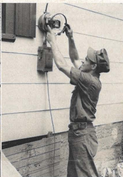
Bill takes a sealing ring loose to remove the meter. He installs a jumper which enables Mrs. Casto to have electricity while the meter is off. Identification tags with the same numbers and the house address are attached to the meter and the jumper.
