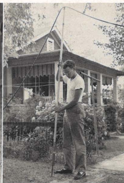
Stewart fastens the cable to a hook at the top of the truck and then to the pole he is shown putting in the ground. This raises the cable off the sidewalk and enables pedestrians to pass safely.
