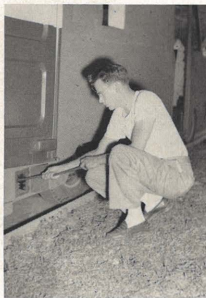
Stewart Foehr of the Charleston meter department pulls the power cable from the truck. The cable will be connected to a special receptacle in the jumper which is placed on the meter socket to maintain service to the home of the customer and the truck.
