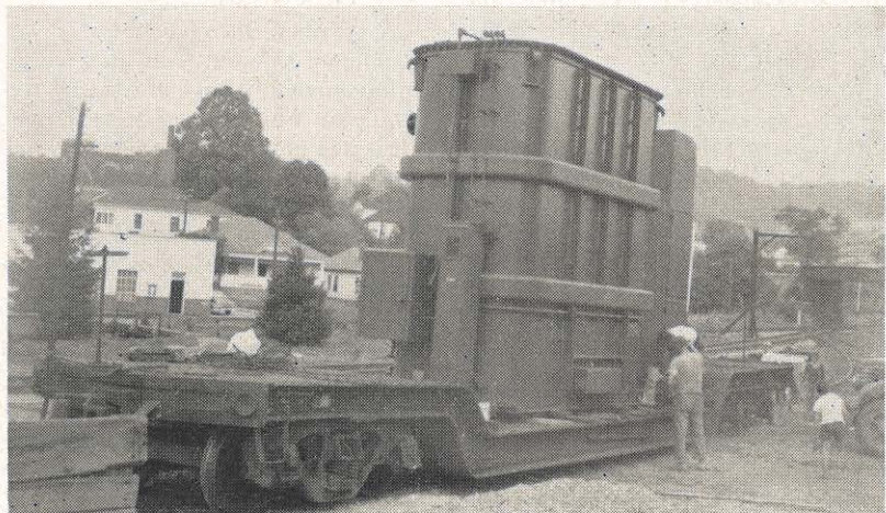
This 30,000 kva transformer has been installed at the Bradley transmission station near Beckley. The Bradley station is rapidly nearing completion and will be put in service soon. It will provide an additional source of electricity to the Beckley area. It is connected to the system by the new 132,000-volt Hinton-Kanawha-Glen Lyn Line.
