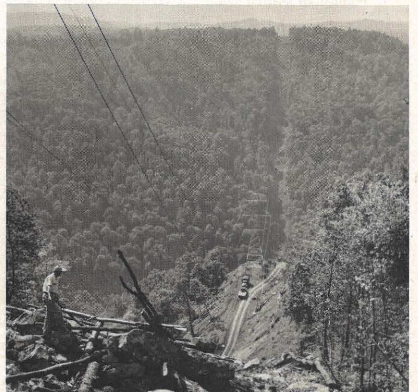
The sagging of conductor begins across the Piney River Gorge near Grandview in Raleigh County. This span is 3,779 feet long.
