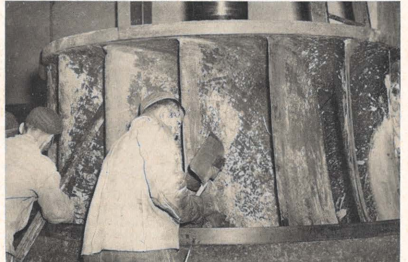
The turbine wheel in the Number One unit at Byllesby Hydro plant gets its first overhauling in 39 years of service.
