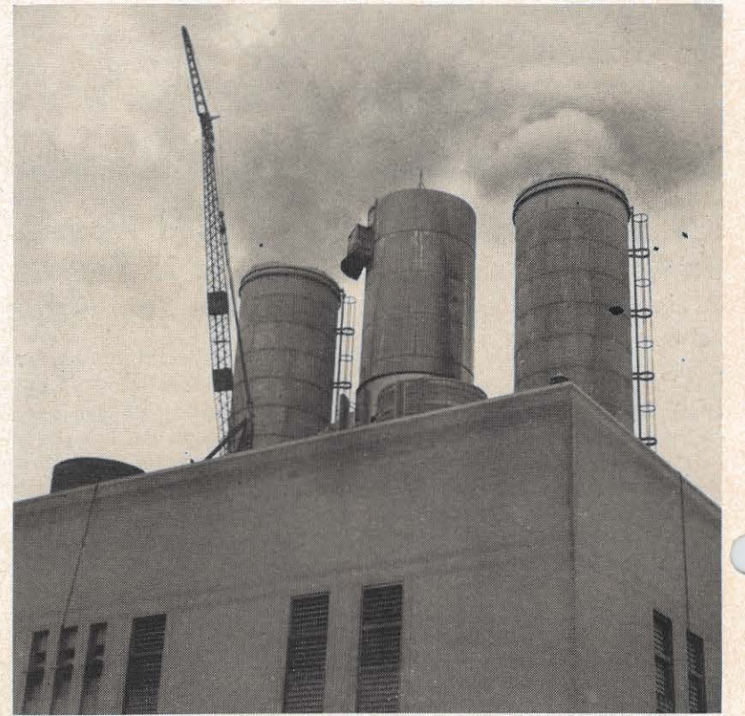
This photograph shows the erection of a new steel stack, center, which will soon handle the flue gas from boiler units eight and nine at the Cabin Creek Plant. This new construction will replace the two existing low-level discharge stacks and carry off gases at high velocity about one hundred and fifty feet above the Boiler Room roof. This alteration is an initial step in a program designed to improve the collection of fly ash. The new stack will be placed into operation sometime in February according to current schedules.
