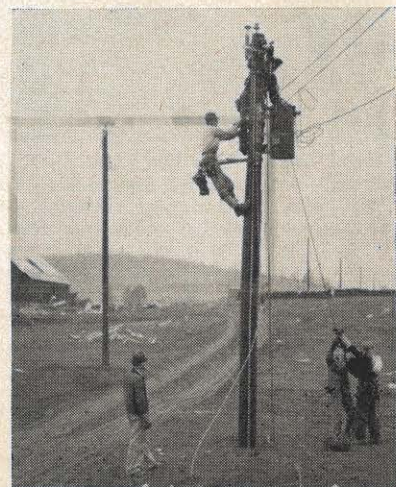
Members of a Kingsport line crew lower a transformer after the 40-foot pole on which it was mounted sank 12 1/2 feet into the ground. Tom Dorton, pictured at the top of the pole, was on the pole pulling in the secondary lines when it sank. Note the slack guy wire in the foreground which was taut before the pole sank. Members of Jack Morrison's line crew, in addition to Dorton, taking equipment down, are J. W. Gilliam, James Johnson, H. G. Brooks and George Smith, on the ground, with Howard Wexler halfway up the pole.
