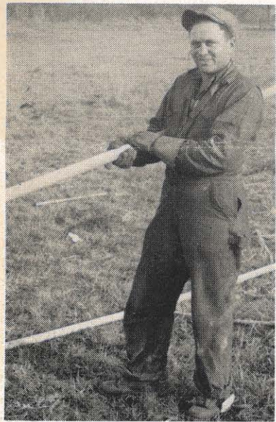
A workman takes a firm hold on the largest conductor ever used on our transmission system. Over an inch and a half in diameter, it has 50 strands of aluminum wire around the outside, then a jute filler and 19 strands of steel wire in the core.
