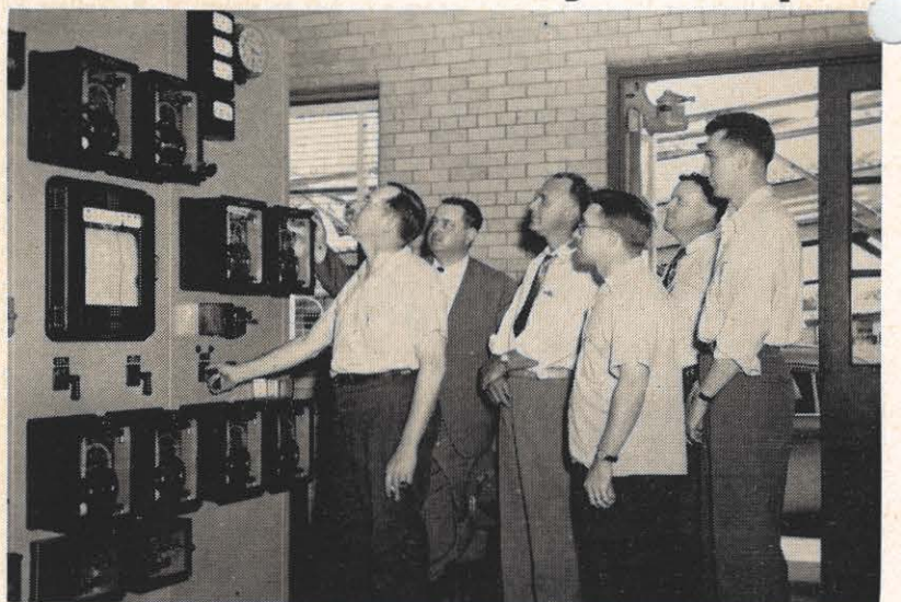
The initial energizing of service to the Vanadium Corporation of America, a new industrial customer on the Appalachian system, was completed May 6 with the closing of a switch by Billy Ribble. Vanadium's 132/13.8 KV main transformer bank is supplied direct by a single 132 KV line from the Sporn Substation bus. Vanadium's ultimate demand is estimated to be about 50,000 KW which will be reached about September 1. Shown above, energizing Vanadium's service, left to right, are: Mr. Ribble, system substation operator, closing the switch; John J. Armstrong and Hansford Buckland, system operating department; M. C. Clark, district superintendent at Point Pleasant, and Messrs. R. E. Freed and J. W. Farley, of the system relay department.
