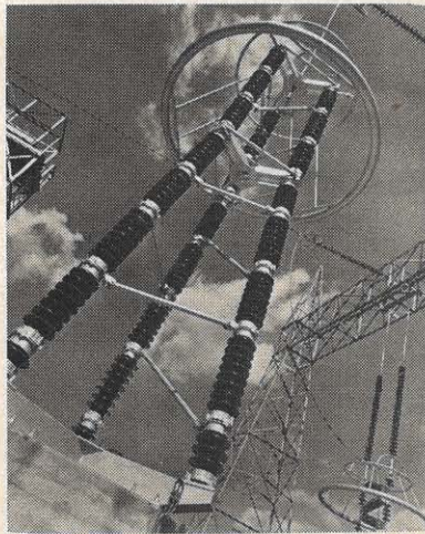
"Modern design for modern living" might be the title of this picture showing the two-story-high pedestal-type lightning arrester. At lower right is a suspended-type arrester. Both are the largest ever built.
