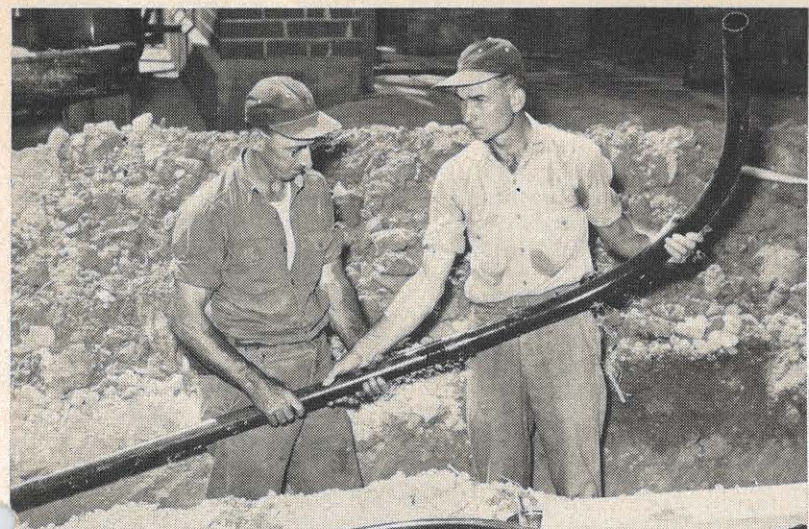
Walter M. Drinnon, left, and Coy A. Arnold, Kingsport Utilities crewmen, hold a section of the plastic pipe with a cemented joint and bend. Because of the flexibility and lightness of the pipe, the men can work in a standing position.
