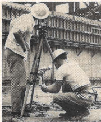
L. Dooley, company survey engineer, sights through the transit as he checks ground dimensions. He is assisted by Ted Law, at the tripod, and Charles Quick, who holds the line at a plant check point.
