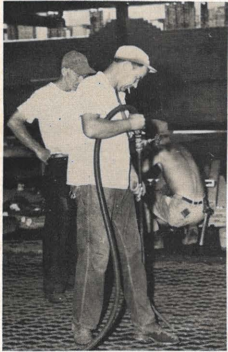
Construction workers clean the "V" decking in the office section of the plant prior to the pouring of concrete.
