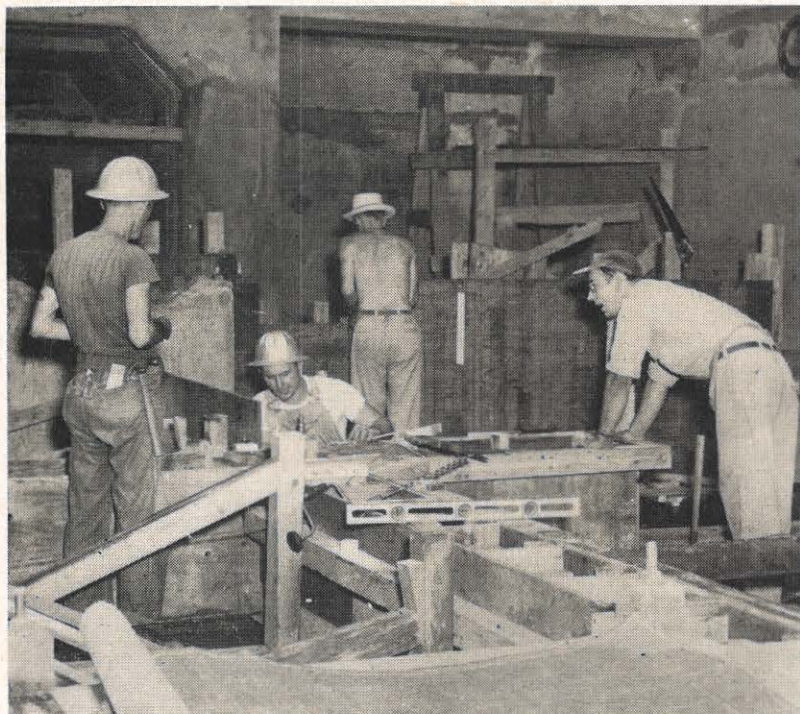
Construction workers are shown building forms for floor drains in the condenser pits for unit No. 1. Note blocked intake tunnels in the background. This will be a source of circulating water for the condenser.
