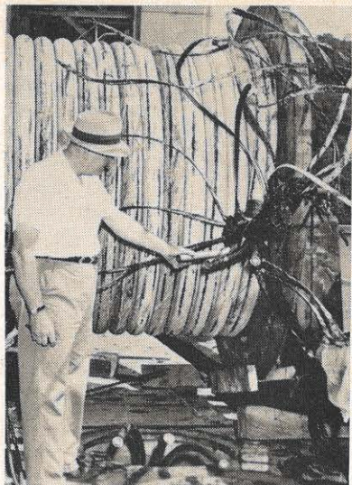
Fred Rotenberry, Claytor plant superintendent, examines the cable used in the vertical section. The wavy wires are the armor.
