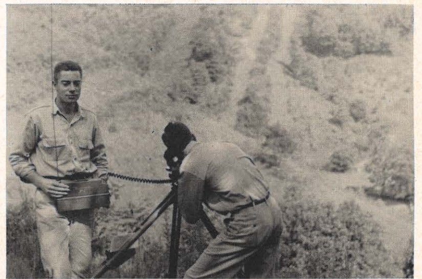
Ralph Damron, transitman on the left, holds the radio while Dorde Picklesimer, transitman, uses transit and radio to sag the conductor. The new line is to the right in the background. Beside this line is the cleared right-of-way for the proposed duplicate 44 kv line. To the extreme left is the old 44 kv line, one mile of which will be removed.
