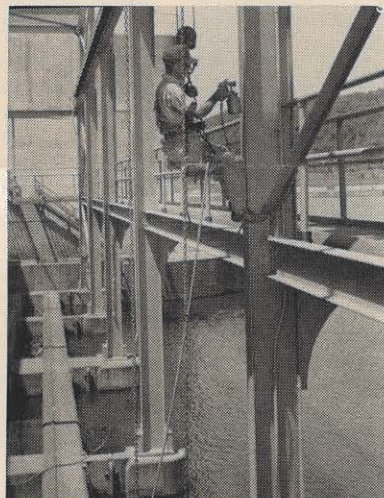
H. E. Brown sprays the new stainless steel paint. This new paint is blue-grey and is expected to give 50 per cent longer service.
