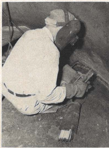
Fred Rymer restores the edge of a turbine blade at Winfield Plant.
