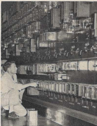
H. R. Miller checks automatic relays while the rest of the crew repair the turbine. The Winfield plant does not require an operator as it is completely automatic.
