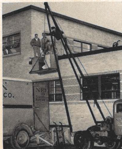
Moving day was helped with the use of this hoist to lift furniture.
