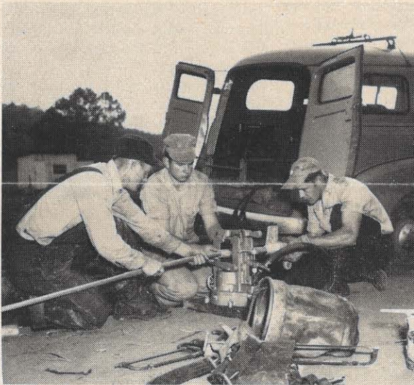
Left to right, C. W. Edmonds, D. C. Harman and Paul Williams install fittings to the conductor after it has been properly cut. The hydraulic ram is a press capable of applying as much as 100 tons pressure to the fittings to clamp them to the conductor. The small high speed gasoline engine, shown in the back of the truck, circulates fluid under pressure to operate the ram.
