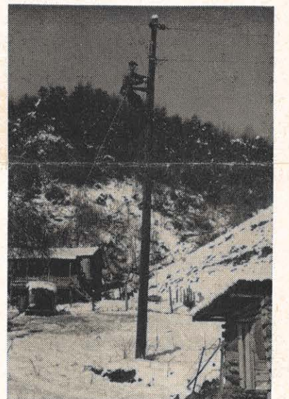
Fred Rosenbaum on pole and Henry Pierce restore service at a rural home where the wire was pulled down.
