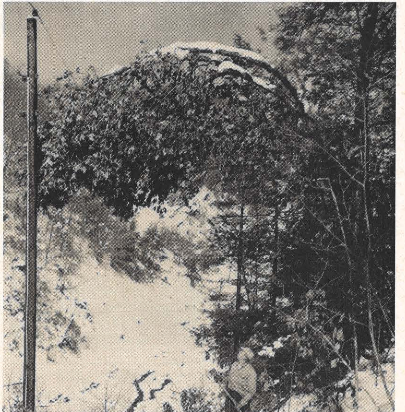
J. M. Orr, substation department, surveys possible line damage before cutting the tree bent under the weight of the heavy snow. Such conditions were general throughout the Abingdon district area.
