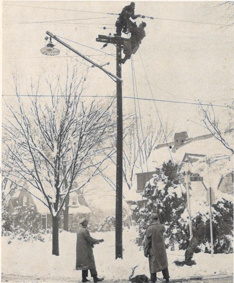
Scenes like this were typical in the Kingsport area as linemen worked long hours to repair the damage. J. P. Smith is atop pole with J. J. Potts below. Groundmen, left to right, are James W. Johnson, George Morrison and Fred Pierce.
