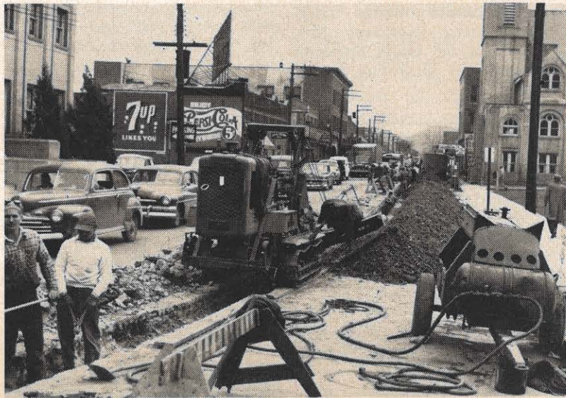
Ditching on Washington Street goes on in preparation for putting in ducts. A total of 275,000 feet of duct will be placed beneath the streets in the downtown area of about one-half a square mile.
