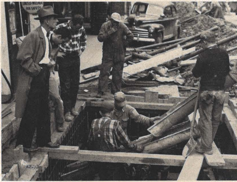
George E. Hervey, Charleston district engineer at left, watches Weikel Construction Company men pour cement for a transformer vault. There will be nine vaults in the underground system scheduled for completion in 1955.
