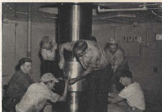
Left photograph, members of the maintenance crew remove the generator shaft coupling guard while disassembling unit number three. Right, a shipyard machinist takes a reading with a twenty-four-inch micrometer during the
