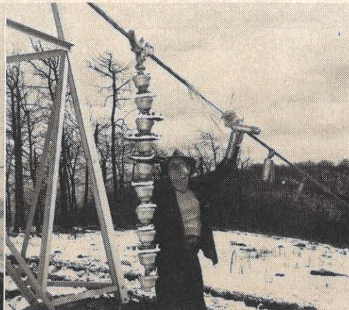
Right, general foreman Roy Doss inspects the damage to the conductor and the insulator.
