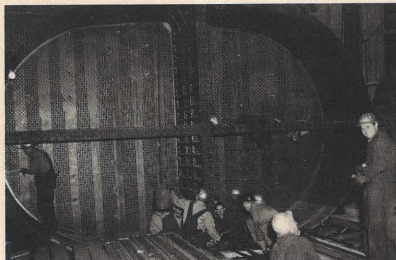
Construction workers put in some of the 13,222 tubes which go into the condenser of unit one. More than 75 miles of the 7/8 inch copper tubing goes into the huge condenser.
