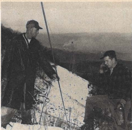
Left, Fred Combs, left, relays sagging operation orders to a distant tower with a walkie-talkie. Right, it is "chow time" on a rush job.
