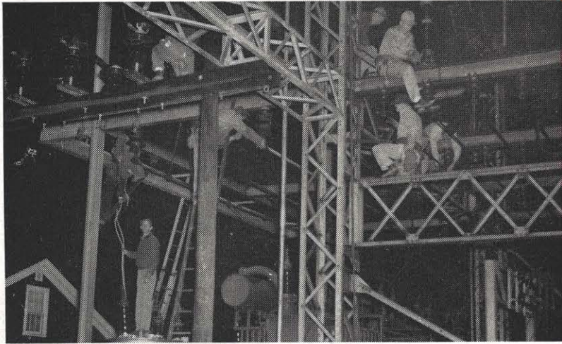
Work begins at Paintsville substation at 5 a. m. No time was wasted as every man did his job. The interruption, planned for two hours, was completed in an hour and 25 minutes when the new 44 kv line went into service.
