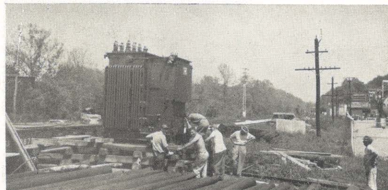
Fieldale district employees unload a 375 kva regulator to be installed at the new 3000 kva Stuart substation. The new station will double capacity in the Stuart area. Pictured are Joel Wilson, Pete Merriman, Junior Nichols, Jim Dalton, Billy Harlowe and Gerald Sanders.
