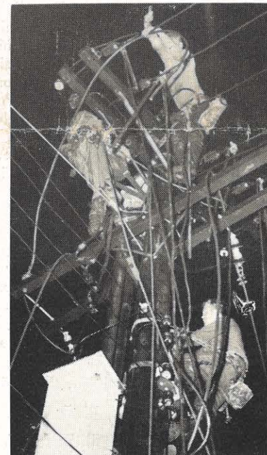
Linemen install a temporary by-pass around the Welch substation which was hit by lightning. Shown on the pole are M. K. Spraker, L. J. Mills, Erle McKinney and H. S. White.
