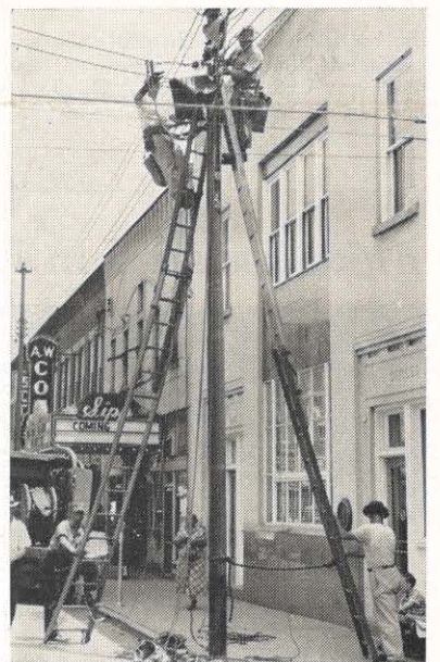
Auburn Helvey and Dennis Clark, Pikeville district employees, work on the changeover in Paintsville to a secondary network. Holding the ladders are Charlie Ratliff, left, and Cecil DeBoard. The business district in Paintsville is being converted from a regular distribution system to a secondary network, requiring replacement of secondary conductors and transformers.
