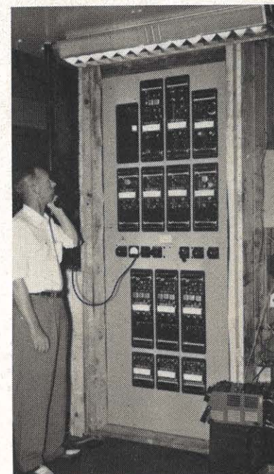
H. A. Clarke, system substation department head, talks to the other terminal at Reusens Hydro near Lynchburg where another electronic relay panel was set up for the tests.
