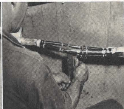
Emery cloth is used on each connector to remove any excess lead and rough spots. The metal shines like new after this operation.
