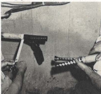
After the cables are cut for the splice, the copper grounding braid is removed to within 2 1/2 inches of the lead sheath and tied off.
