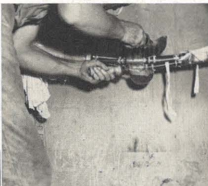
The exposed cable cleaned, lead is poured time and again over the connectors. This seals the splice and sweats out moisture.
