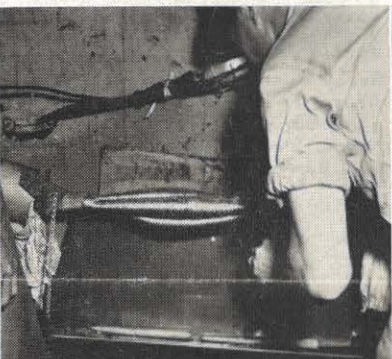
Before these three wires were covered with this copper braided grounding tape, boiling oil was poured over all exposed parts to remove moisture and foreign matter. Each connection was brought up smooth with the rest of the conductor with narrow tape, then wrapped with oil tape—a very tiring and lengthy process.
