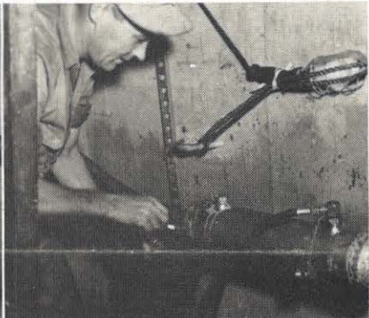
The sleeve is under air pressure as this soapy solution is painted on to be sure there are no leaks. The sleeve is then filled with a hot tarry solution. After the solution cools, the plugs are put in place to finish the job. Although this splice took eight hours to complete, some of the major splices take longer.
