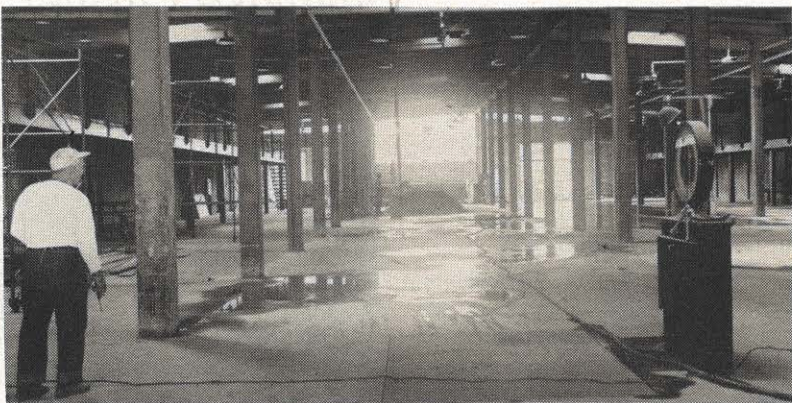
Roanoke stores building is rounding into shape as the concrete floor and the mezzanine storage areas at each side of the building are complete. When this picture was made September 18 the wall at the far end of the building was almost finished.
