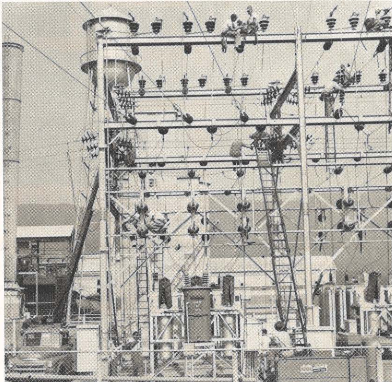
Insulators are switched at the substation which furnished power to the Lone Star Cement Corporation. The men working on the substation were in teams and distributed over the structure to reduce the danger of falling objects.
