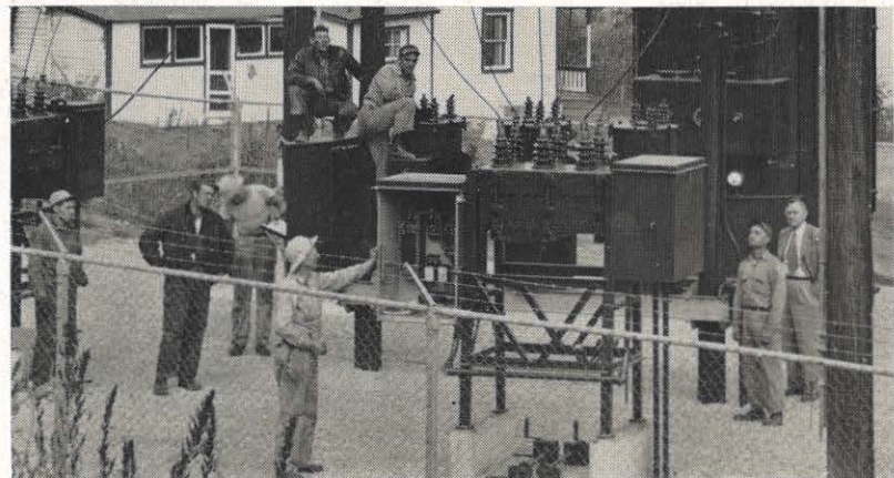
Crews make a final check before energizing the Barrenshe substation in the Sprigg district. Located near Freeburn in Pike County, the station replaces an old switching structure and has 2,500 kva capacity. It will serve several towns in both the Williamson and Sprigg districts as well as rural lines.
