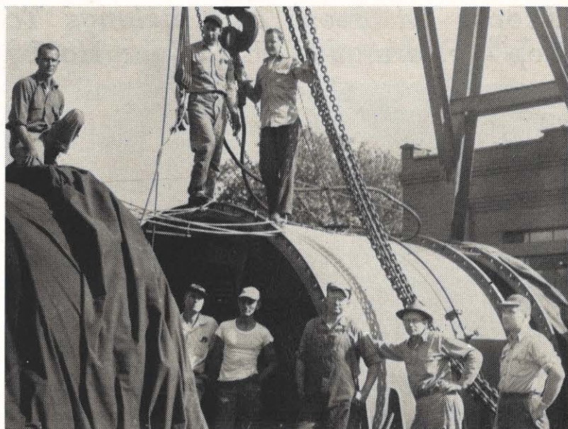
Scarbro substation crew members "take a break" as they give the 15,000 kva condenser a complete overhaul. The reconditioning is done every five years when every part is taken down and cleaned, greased and replaced. Helping on the Beckley district substation job was J. E. Matthews, foreman from the Charleston substation department. Pictured from the left on top are L. C. Jones, J. C. Keaton and Richard Patterson. Below, from left: J. P. Hughes, J. B. Richmond, A. R. Allen, L. C. Mollohan, foreman, and R. J. Pinnell.
