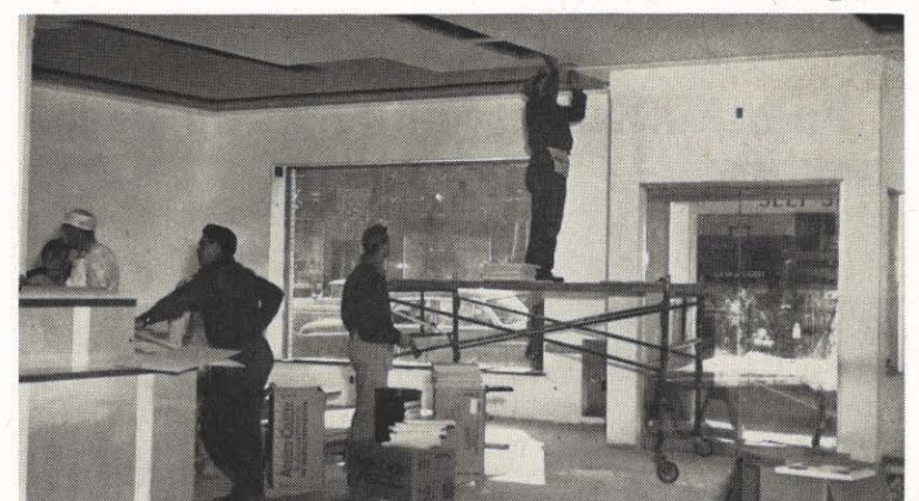
With occupancy expected in two months, the Pulaski office building is being given the final touches. Here, workers apply acoustical board to the ceiling of the main lobby. Lighting fixtures are being installed, while painting, installation of air conditioning and finishing of floors will get under way soon. With the completion of the floor in the vault the telephone company can install their equipment.
