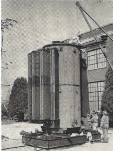
System transformer repair crew members under Foreman R. L. Lewis mount radiators on a transformer from the No. 1 20,000 kva bank at Holston substation in Kingsport. Work on the bank, undergoing general repairs, re-gasketing and painting is expected to be completed next month. Frank Noe and Jim Ward of Holston station assisted with repairs. Members of the system substation department on the job were J. E. Glover, J. E. Moore, K. D. Ferguson, W. M. Connor, C. E. Carter and L. C. Woodford.
