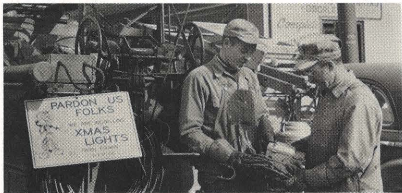
Frowns on Bluefield motorists' faces turned to smiles after they passed the truck that was temporarily blocking traffic. Reason for the change of attitude was the sign pictured above with Reddy Kilowatt which says, "Pardon Us Folks, we are installing Christmas lights." The signs were used on the back of service trucks while the lights were put up. Bob Crowder and Charlie Hedrick of the Bluefield line crew are shown examining one of the switchboxes before it was installed on a Christmas street light circuit. The lights were turned on Thanksgiving night.
