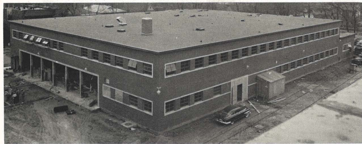
Brickwork is completed on the Huntington service building, expected to be finished in February.
