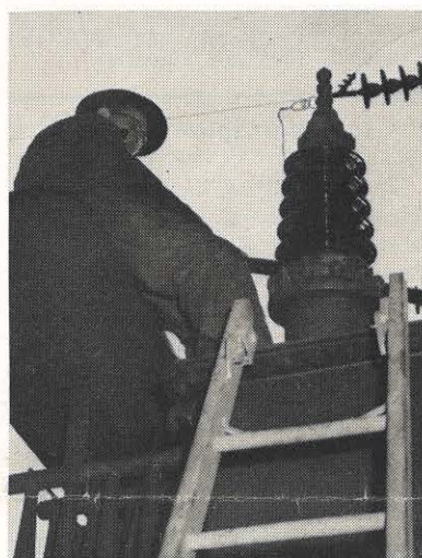
A close-up of the patient and nurse. L. C. Mollohan grins as he hears the test engineer call that the transformer's illness has been diagnosed. Surgery is the recommendation—with the doctor's promise that in "a few days you'll be humming like new."
