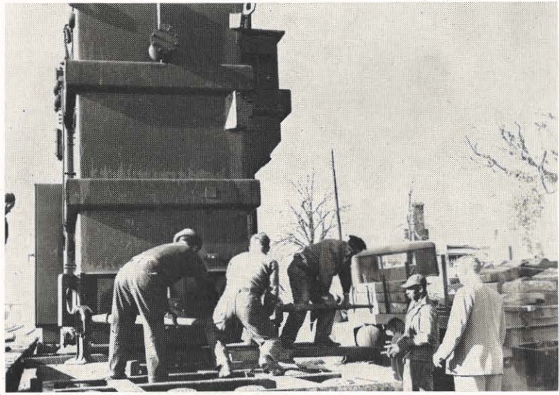
Men unload the 65,000-kva transformer which will be installed at the new 132,000-volt transmission substation near Wytheville.
