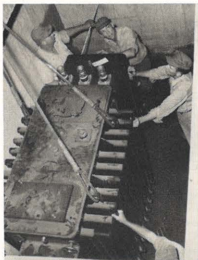
Taken during the early part of work on the underground system, this photograph shows, from the left, Charles Kelley, Steve Didier and C. R. Street working a transformer into position before placing it.
