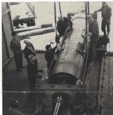
FIFTH: The field has been moved from the turbine room and secured in a cradle. In this view the field is about to be lifted to the flat car.
