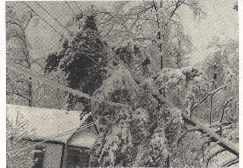
TOP: This Ashland scene shows some of the troubles faced by line crews. No one was hurt in this tangle of utility wires which Ashland crews are shown repairing. (Photo Courtesy "Ashland Daily Independent")
