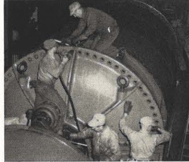
FIRST STEP: Workers remove bolts from an end shield of the generator with a pneumatic wrench.
