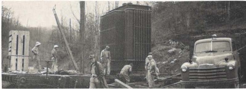
The Welch district station maintenance crew is shown unloading a Westinghouse 7,500 KVA, 88,000 to 33,000 volt transformer at Faraday station for installation. The new transformer replaces a 88,000 to 13,200 bank now in the station. Weight of the new transformer is 67,650 pounds. Members of the crew are, from the left: J. P. Sutphin, O. L. Lamastus, Ralph Slade, W. C. Sexton, G. N. Rutherford and F. L. Lineberry.
