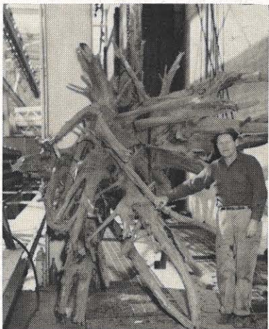
This tree stump was the cause of real work by G. V. Loveday who had to get it out of the trash racks at Marmet hydro plant. Trees form a large part of the debris caught in the rack.
