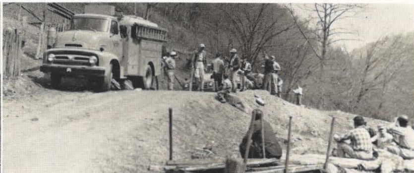
The job is finished within the time scheduled for the outage. Men came down from opposite hills, carrying rope and equipment, to meet back at the trucks. Here, lunch is being served to men who are ready to eat after having worked long and hard since that early Sunday morning breakfast at 4 o'clock.
