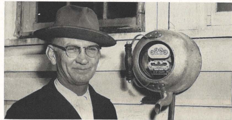
"It ain't so," said Joe Lewey, Pearisburg area serviceman in the Bluefield district, when he saw this meter housed in a tea kettle. But it was. Seems a customer was doing a major remodeling job on his house and accidentally broke the glass meter cover. In order to keep the rain out of the meter until its cover could be replaced, the customer cut out the bottom of an old aluminum tea kettle and fastened it as shown above. It does the job nicely.
