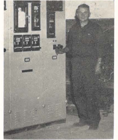
C. T. Smith, Niagara Hydro plant operator, stands beside the new automatic controls just completed at the plant.
