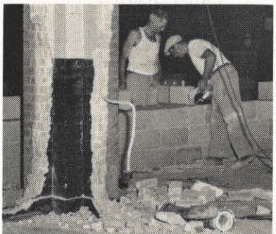
Workmen lay cinder blocks for partitions in the remodeled Charleston meter building. Jagged edges in the foreground are remains of old partitions.
