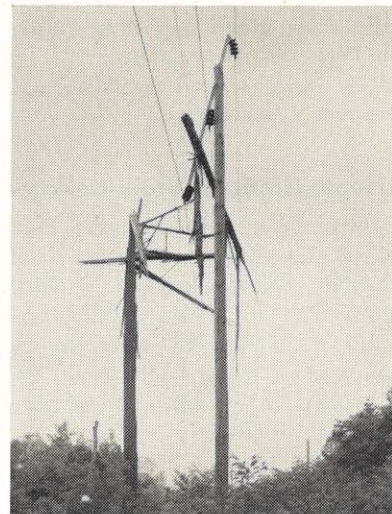
Lightning can play havoc with electrical facilities, as shown here when a bolt hit the 44,000 volt Prince to Layland line. One of the poles was hit directly but the steel arm swung into a near-vertical position, eliminating an outage. Pieces of the structure hit directly were found almost a mile away. A customer reported the damage which was soon repaired.
