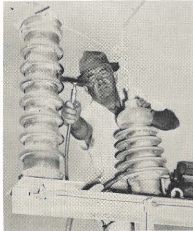
D. R. Whittaker, Giles County area supervisor, uses a scratch wheel on some insulators that had to be cleaned on the job.
