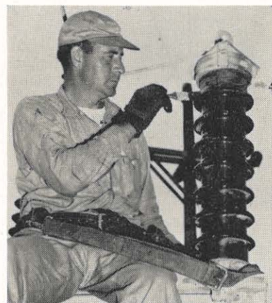
David M. Davis, Giles County line crew working foreman, perches in a high place to apply a hot wax solution to insulators.
