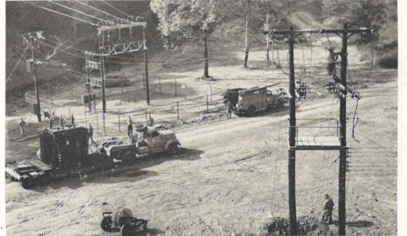
Arriving at the site after its trip over the mountain, the transformer is ready to be installed. Despite a 30-minute delay, the entire job took little over half the time provided for the interruption.
