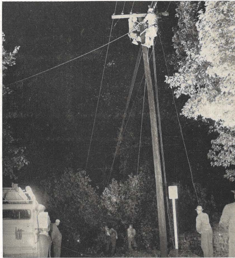
Trouble from Hurricane Hazel was left throughout the Roanoke division. Here, C. E. Firebaugh's crew works to restore service Friday night at 13th street in southwest Roanoke while city workmen cut the fallen tree off lines.
