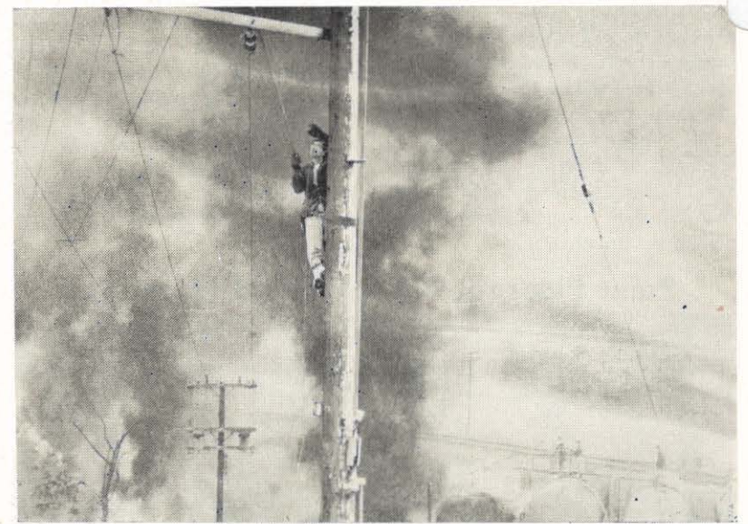
Flames from a $75,000 oil plant fire roar near Forrest E. Phillips, but the Pikeville district general serviceman calmly disconnects the three-phase line serving the plant. Action took place in Shelbiana recently when fire struck the Gulf Oil bulk plant, destroying buildings, storage tanks, gasoline, oil, auto parts, a railroad tank car and several utility poles. To add to Mr. Phillips' danger it was snowing when he scaled the pole, as evidenced by the snow on side of the pole and the haziness in the background. Firemen spray a storage tank in the lower right hand corner to prevent further damage.
