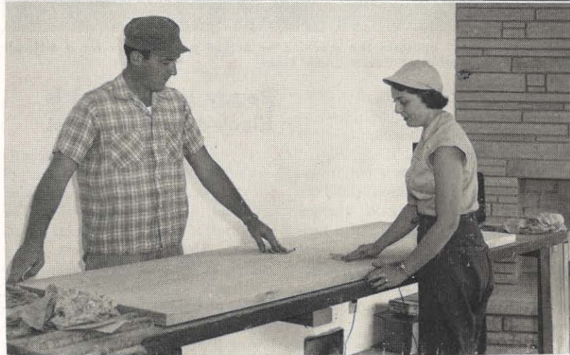
The house in the top picture is the result of work like that being done in the bottom photograph. The house belongs to James E. and Doris J. Fleenor, Abingdon district employees. The two are doing almost all the work in construction of the house and hope to finish next year.
