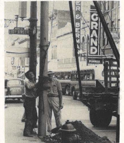
"These poles will last for at least 40 years." That's the remark H. W. Proffitt, Lynchburg line foreman, on the right, heard from a company official 40 years ago when he helped install them on the city streets. And Mr. Proffitt can vouch for the amazing prediction as he helps A. L. Ward, lineman, remove the poles. It's all part of street light modernization in Lynchburg, exactly 40 years after the official's uncanny remark.
