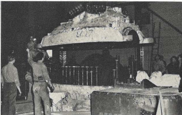
Away she goes! Being careful to keep the casing precisely level to avoid damage to the internals, it is hoisted clear, exposing one end of the turbine rotor.
