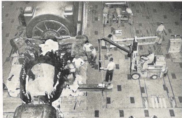
Power equipment and manpower join forces as the actual repair work begins. The rotor, in the center of the picture, is covered for dirt and damage protection.
