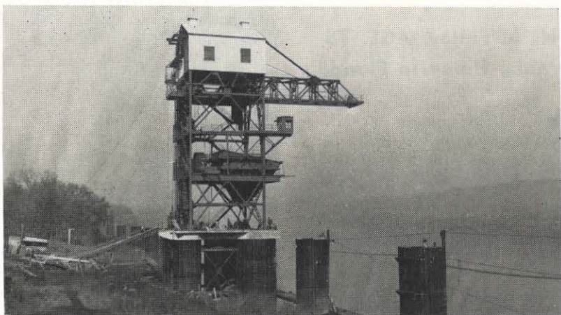
Almost completed is the stationary barge unloading tower at Philip Sporn plant. The tower is part of the major improvement being made to the coal unloading docks. The tower, 100 feet high and standing on four piling cells 33 feet above the normal river level, has a gantry crane bucket operating from the cantilever beam and handling 12 tons of coal each trip. It will unload coal at the rate of 1,200 tons per hour. The tower also has a man lift for operating personnel. Other improvements to be made include conveyors from the unloading tower to a stand pipe in the coal storage area and conveyors from the stand pipe to the conveyors leading to the plant.
