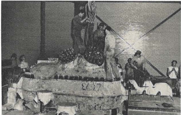
Workers place slings in position for lifting the top casing. Insulation has been removed from the casing, the steam leads disconnected and stud nuts removed.
