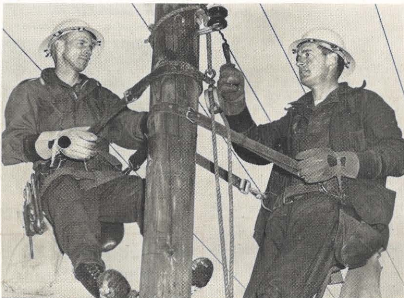
It takes energy . . . to keep up with growing demands. It is estimated that by 1975 the demand for electrical energy will increase by 250%. Linemen like I. H. Mace and R. C. Childress, Abingdon district, will help meet that growth.
