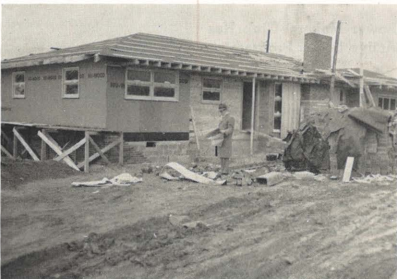
New families need new homes . . . and everything that goes in them. Since 1950 we have built three million new homes—not enough. M. C. Simpson, Kingsport commercial manager, looks at blueprints for another electrically heated home.
