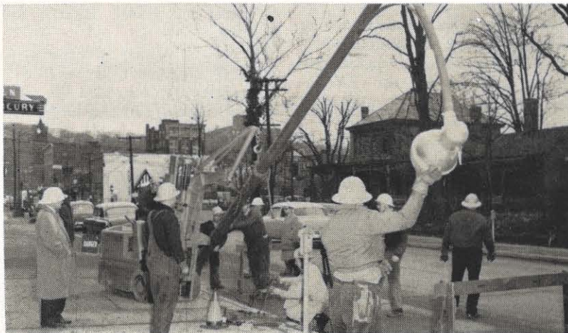
This fork lift truck recently went to town in Charleston, helping to install street light standards for the underground electric system. As you can see in the picture, the fork lift can go in spaces where traffic and parking conditions prevent the use of a line truck and the conventional A-frame. Then, too, it can and does run on the sidewalk. Shown above, from the left: E. H. Braid, distribution supervisor, Lloyd Post, lift operator, T. K. Rhodes, Paul Hull, Curt Willis, John C. Frazier, safety supervisor, Kermit Fisher, engineer, W. H. Barker, kneeling, Robert Jones, back to camera, Leland Price, line foreman, and R. H. Taylor, back to camera.
