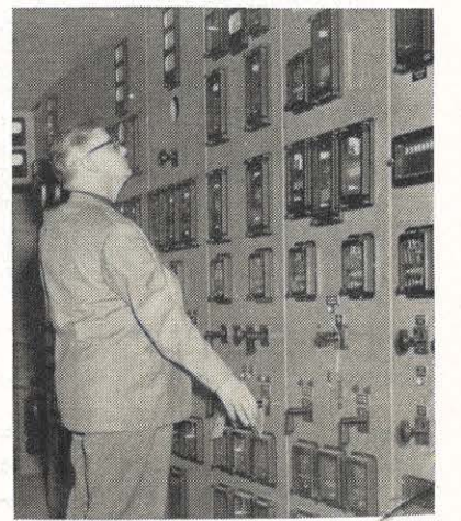
History was made in Appalachia when Lindsey B. Ferguson threw the switch for the first sleet melt test on 330,000 volt lines. The assistant chief system substation operator at Sporn station is shown beginning the test.
