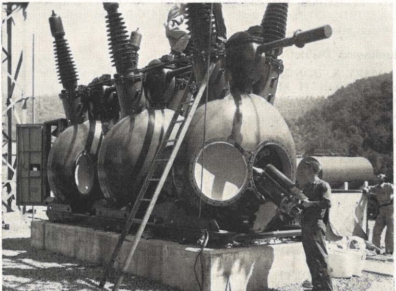
Workmen install interruptors on a new-type oil-circuit breaker at Kanawha River plant. This was the first of 10 of these 138 kv lenticular-tank breakers to be installed. These 10 million kva breakers made by GE are being used to replace present breakers rated at 5 million kva. The replacement program is scheduled for completion this year at Kanawha River plant. In the future the manufacturer plans to ship the breakers completely assembled, with only connections and adjustments needed before they can be put in service.
