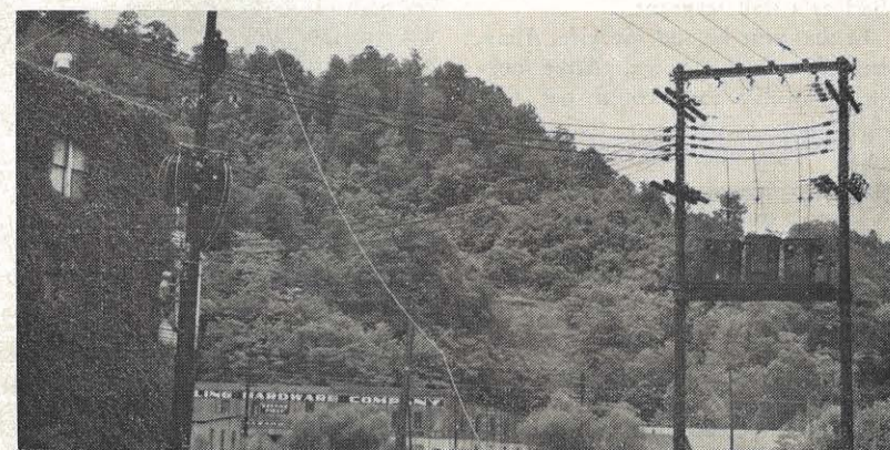
"In with the new and out with the old" takes place early Sunday morning as Hazard linemen convert the town's distribution system. The old transformer bank at the right in the picture was replaced with the cluster bank on the pole at left. At the top of the pole is Neldon Whitaker and below the bank is Wesley Yonts. Fred M. Skaggs is on the roof. Revamping the business section meant installing new circuits, new and larger transformer banks and extension of larger services to customers. This work was done during the week with the change-over made early Sunday morning with service remaining constant.
