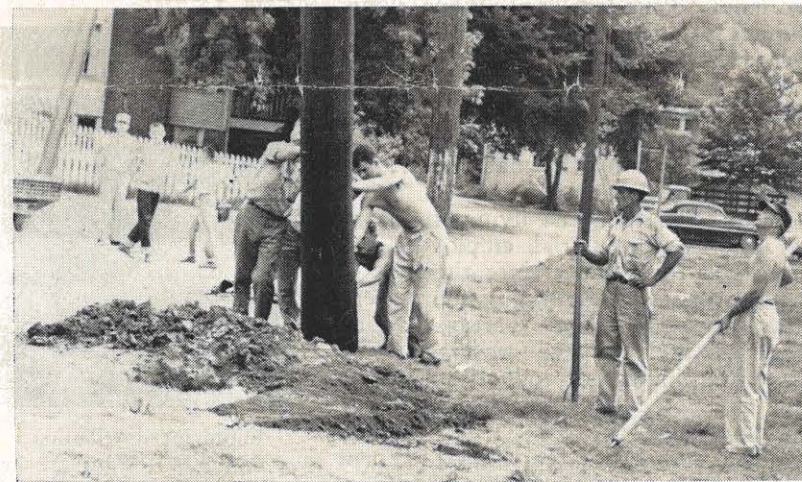
Moving a pole over the hole with an A frame at the Little League field are several Pikeville employees. Identifiable in the picture are from left: Raymond Scott, Bill Zoellers, L. R. Newsom, James Burke and L. M. Newsom.
