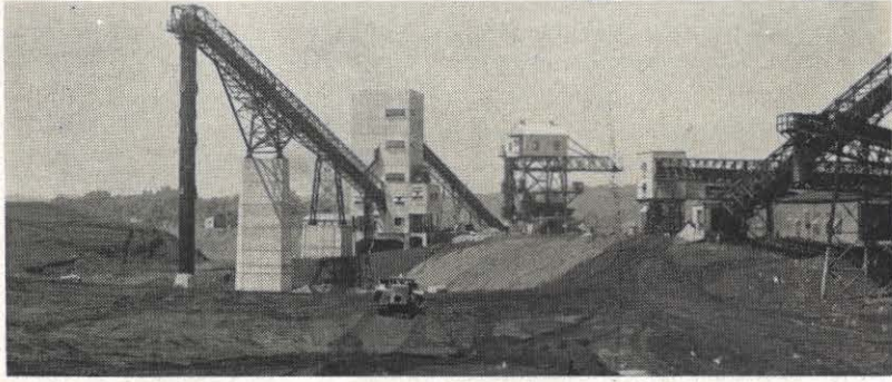
This photo shows the new coal unloading system at Philip Sporn plant. The unloading tower at rear stands 100 feet high and moves the huge bucket which holds 12 tons of coal.
