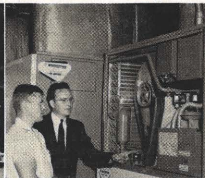
RIGHT: Robert Porter, market manager at left, looks over a heat pump unit with Otho J. Bragg, Welch district commercial sales representative. An important point about the heat pump and the market was pointed out by Sidney Peery, Acme president, when he said, "While we are using all-electric equipment, we are also using coal—about the equivalent of 200 tons per year, coal by wire."
