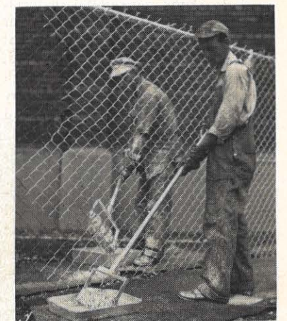
Rollers help these Cabin Creek plant employees do a real paint job. They painted over 4,000 feet of 7-foot fencing in record time. G. W. Abshire, near side, and E. E. Crist, also of the labor department, used the rollers to cut painting time by 40 per cent. A third man touched up spots with a brush to complete the job.
