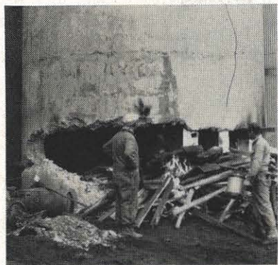
Flames lick at the 12 by 12 oak timbers supporting the stack after its base has been chipped away. This was done, much as in felling trees, so that the stack would fall in the proper direction.
