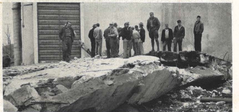
"It mashed flat" and "It crumbled up like a hollow tree" were comments heard after the dust had settled. Kingsport Utilities line crew members look over the remains of a Kingsport landmark. At 12:50 Saturday afternoon, December 3, ahead of schedule, the first tower came tumbling down. Five days later, at 12:15 p. m., the other was felled. A New York demolition crew was contracted for the work.
