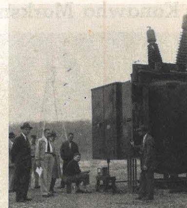
A. C. Rogers, assistant system station superintendent, is at the controls during recent oil circuit breaker tests at Philip Sporn station. In the left foreground is Jack W. Kepner, assistant superintendent of system operations. Next to him is Otto Naef, AGE circuit breaker engineer, who was in charge of the tests.
