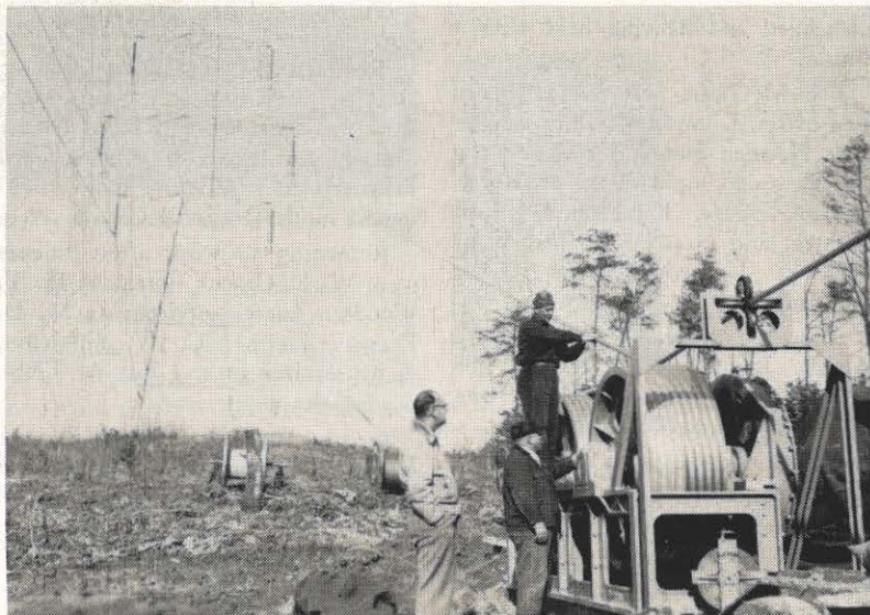
The 330-kv Sporn-Kanawha line gets a close inspection from three employees in the left picture. Shown are Hansford Buckland, chief system substation operator, and W. F. Sage, on the ground, and W. A. Jefcoat, standing on the
