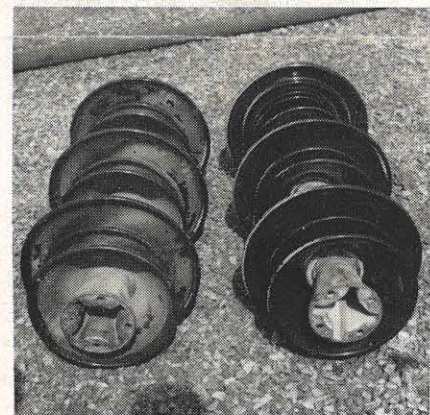
LEFT: Before and after. The insulator at left needs cleaning and the one at right has been washed hot, showing how effective the new method is. RIGHT: These are the men who wash insulators hot. All members of the system transmission line department, they are experienced in their work, which began in 1945 under J. Bradley Doss, system transmission foreman until January 1, 1954. When he
