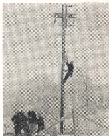
Repairs are being made to a toppled crossarm. Beckley crews worked long hours to restore service after the Friday 13th snowstorm.
