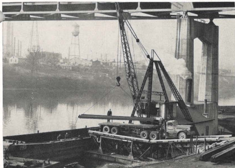
This transfer of steel for Glen Lyn plant from barge to truck marks a new chapter in West Virginia's transportation picture. This was the first heavy freight load to use the two-step movement which Charleston Chamber of Commerce officials said focussed attention on what might become a substantial addition to the state's traffic pattern. The steel beams were produced in the U. S. Steel's Pittsburgh mills, loaded on barges and brought down to docking facilities at Reed. Trucks took the steel beams over the Turnpike to Princeton and over another road to Glen Lyn. The shipment spotlights the combination of water and highway for heavy freight between the Detroit-Cleveland-Pittsburgh area and southeastern points on the Atlantic Tidewater, Chamber officials said. (Photo by E. T. DuMetz, Courtesy Gazette)
