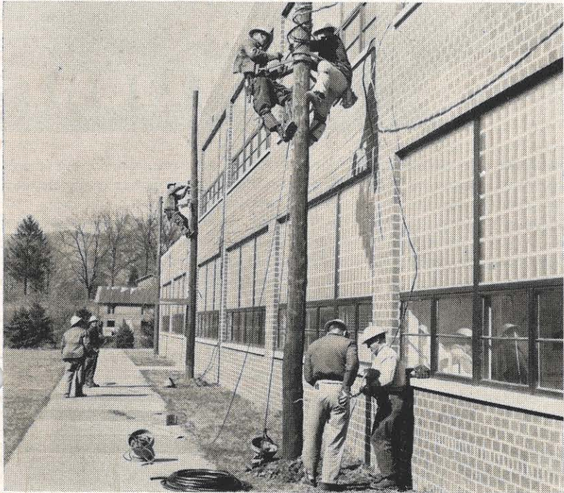
Bringing temporary emergency service to the Pearisburg school was a hurry-up job. Here the Narrows line gang attaches service to the temporary poles. On the ground from left are D. R. Whittaker, area supervisor; Charles Peirce, lineman; H. B. Boyd, lineman; and David Mann, groundman. On the poles are from left J. D. Butler, lineman; W. B. Rasnake, lineman; and W. H. Conner, Jr., lineman.
