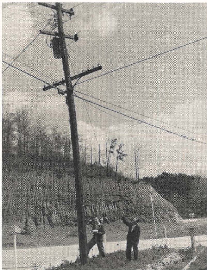
Checking a "dual-purpose" pole are employees of Appalachian and the Chesapeake & Potomac Telephone Company of Virginia. K. D. Cox, left, Roanoke district engineering aide, checks the section map while D. W. Ash of C&P checks the attachments.
